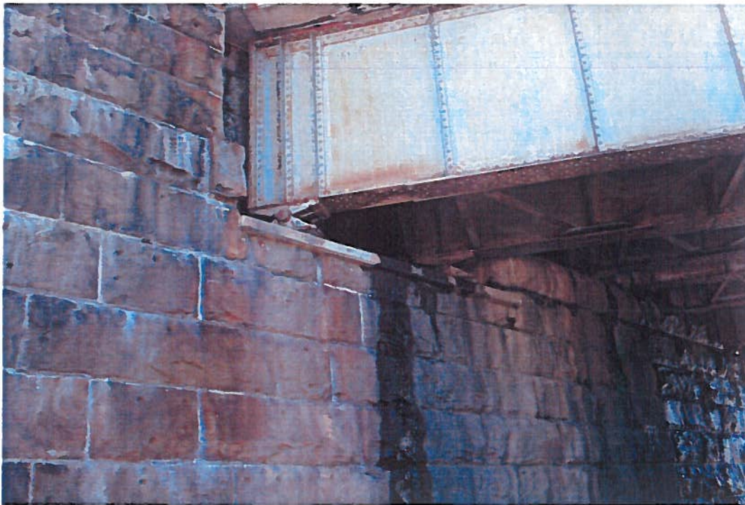
Abutment chop-down, capping & leakage at Juniata Street
