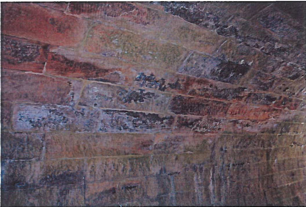
Leaching & discoloration within Freedom overpass
