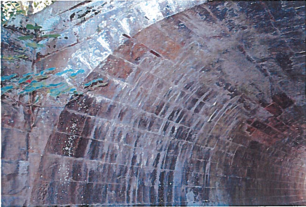
Leaching & discoloration within Freedom overpass, at north end
