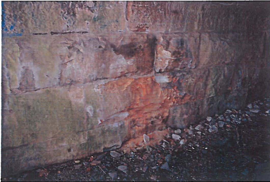
Leaching, discoloration & deterioration within Centennial overpass
