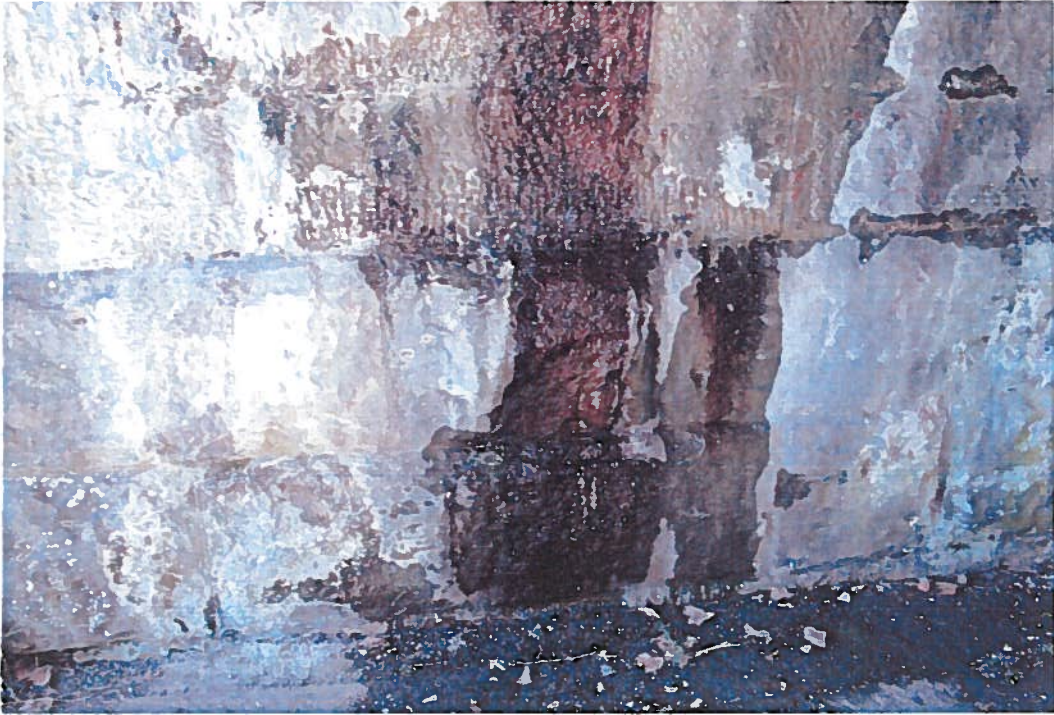
Leaking & leaching within Centennial overpass
