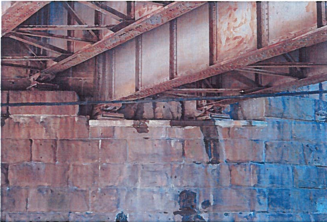
Abutment chop-down, capping & leakage at Juniata Street
