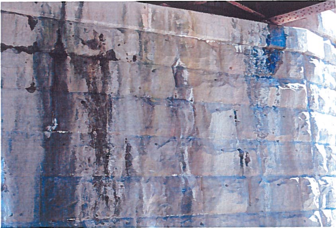
Leaching & deterioration at Stokes abutment
