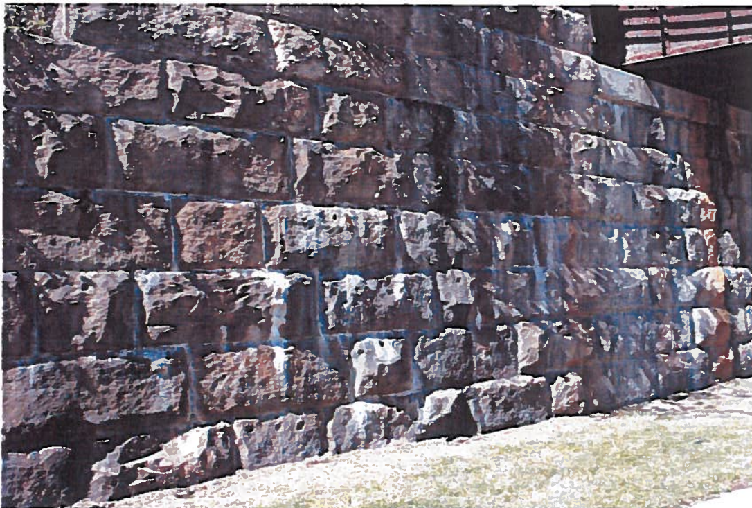
Leaching & leaking at Stokes Street abutment
