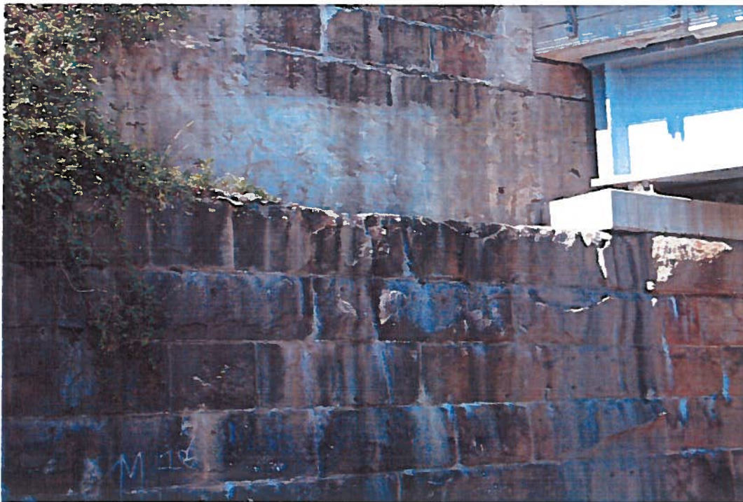
Patching & leaching at Adams Street
