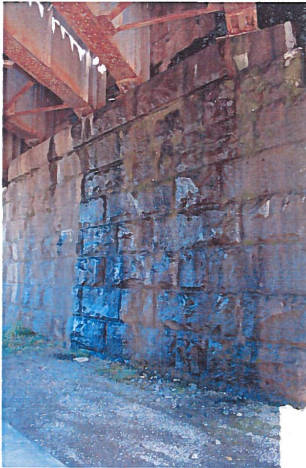
Abutment leakage, deterioration & discoloration at Juniata Street
