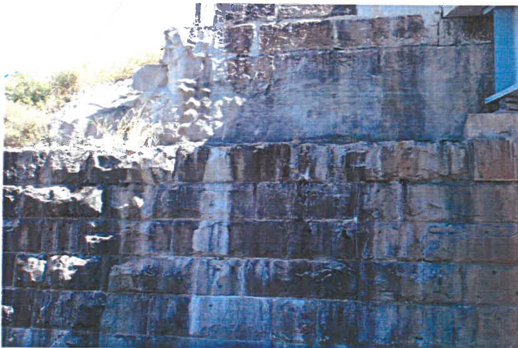
Severe abutment stone deterioration & leaching, with major modifications at Adams Street
