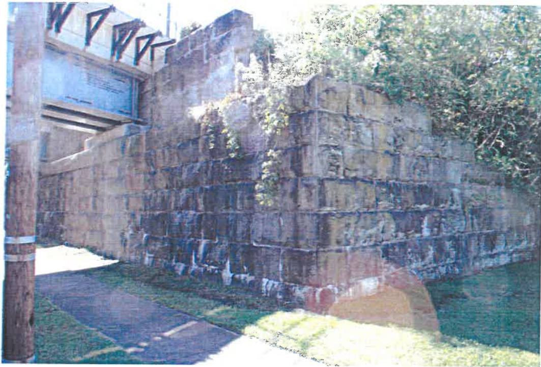
Chop-down modifications, leaching & deterioration at Adams Street
