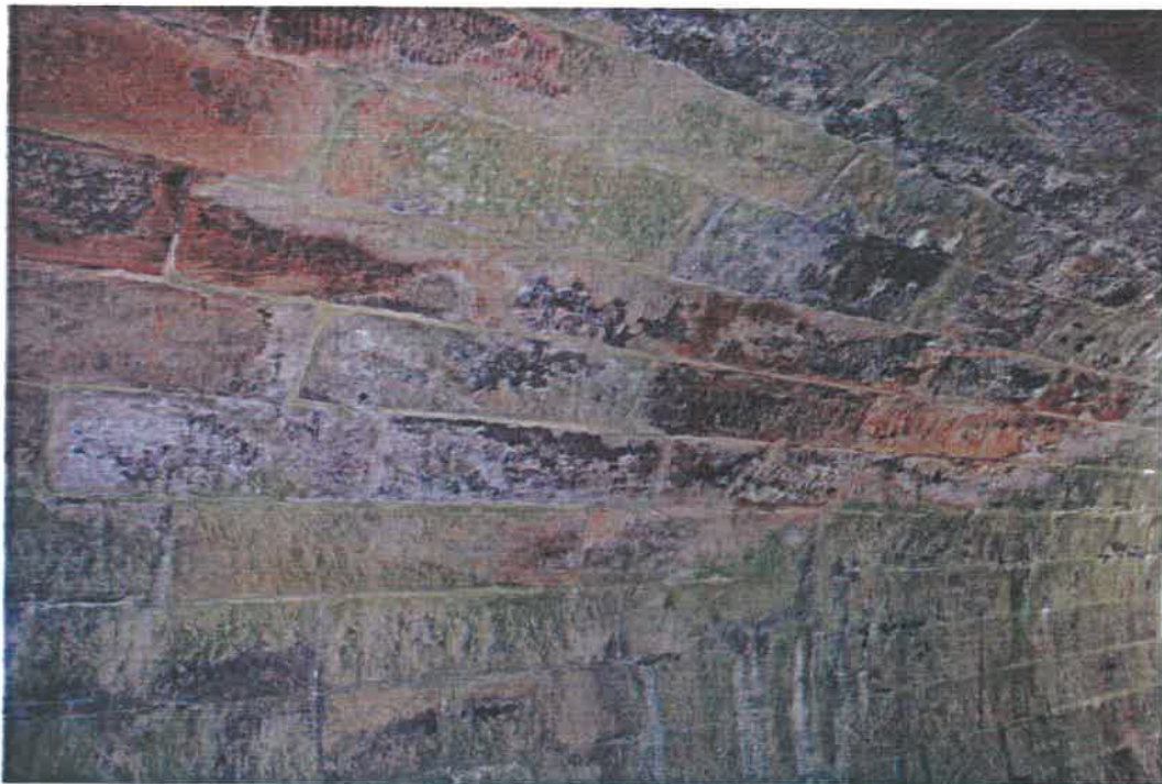
Leaching & discoloration within Freedom overpass
