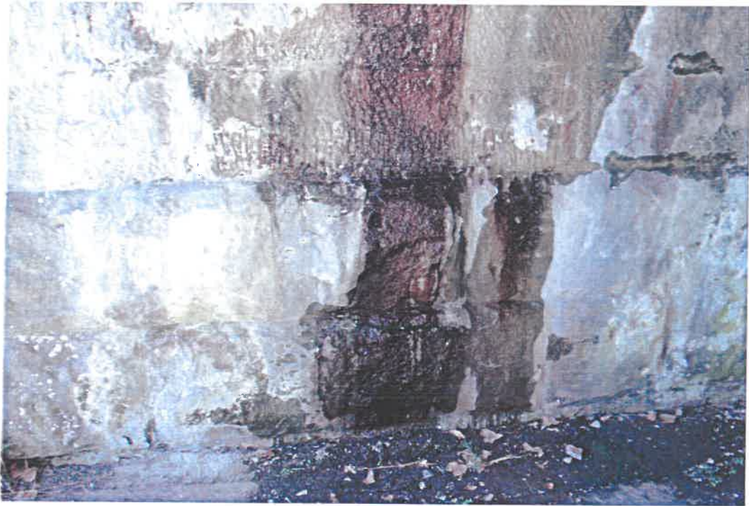
Leaking & leaching within Centennial overpass
