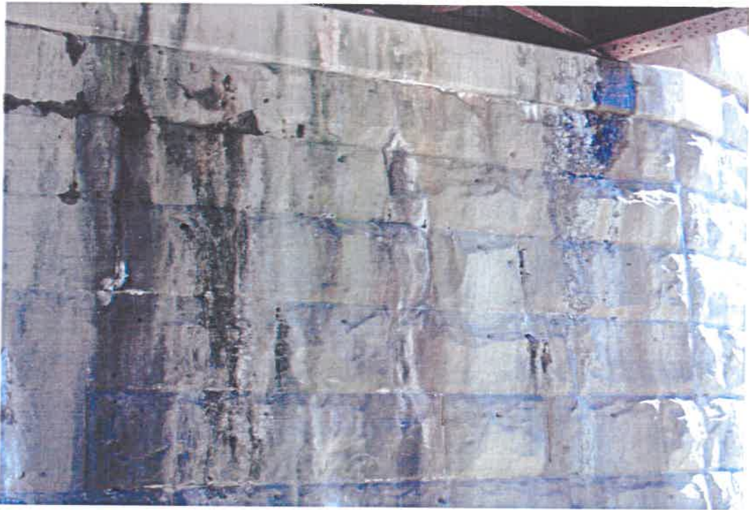
Leaching & deterioration at Stokes abutment
