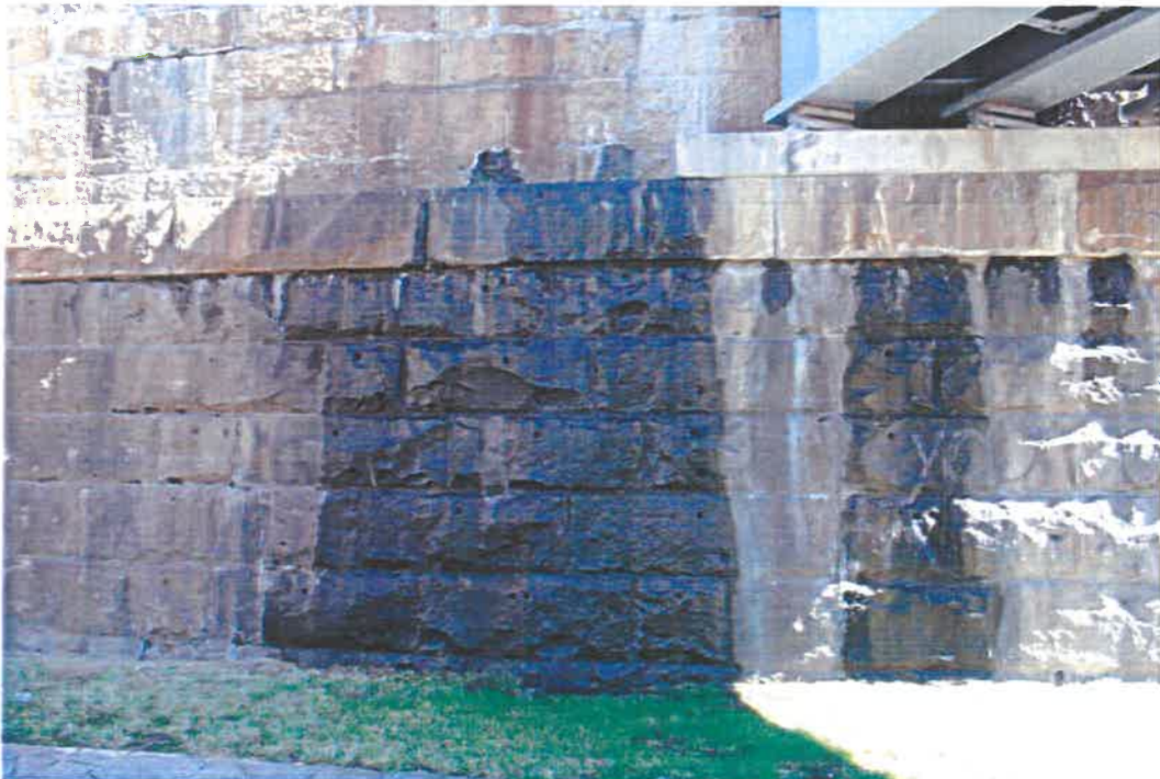
Extensive leakage & leaching at Adams Street
