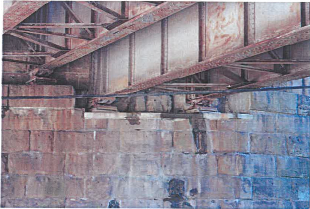
Abutment chop-down, capping & leakage at Juniata Street
