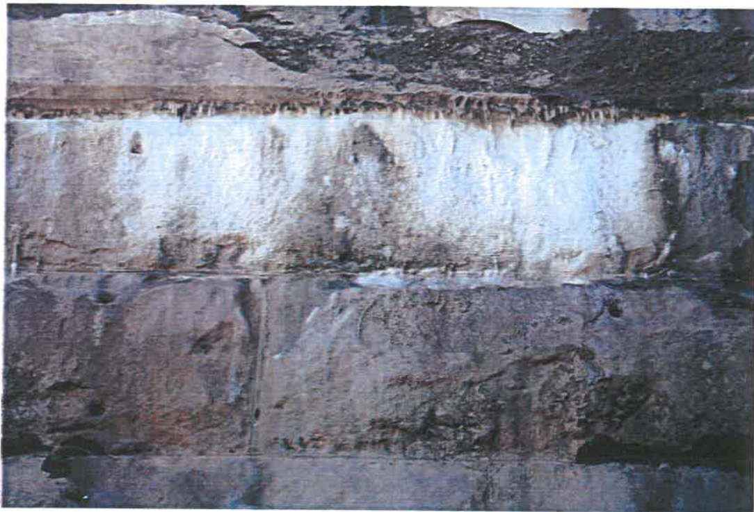
Leaching & deterioration at Stokes abutment
