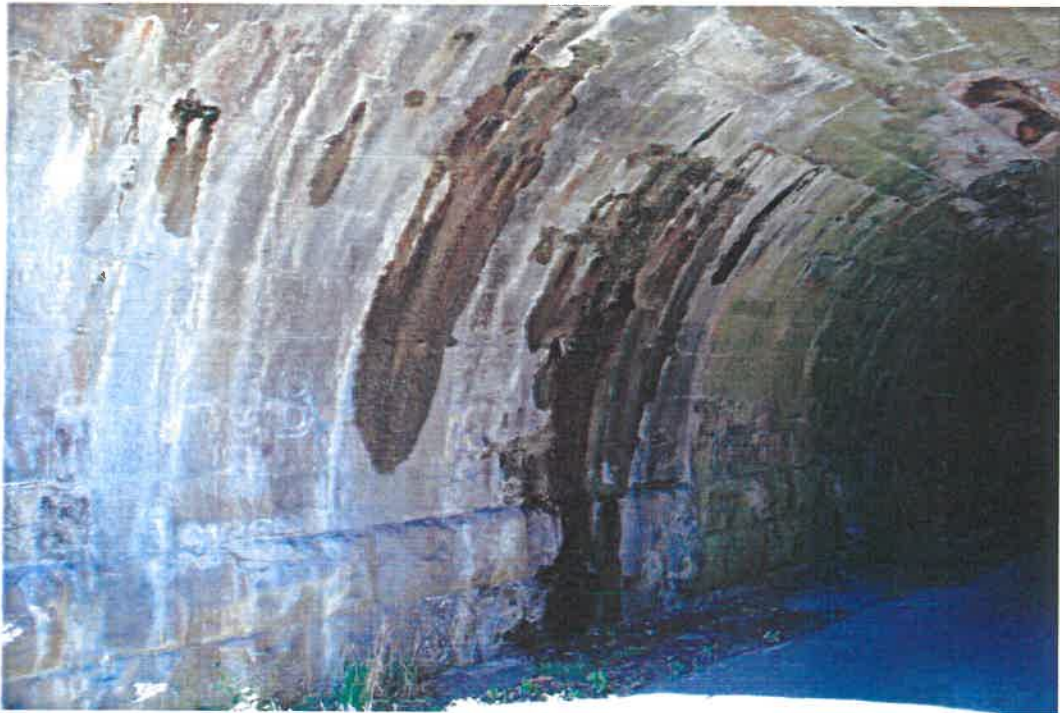
Leaching & leaking within Freedom overpass
