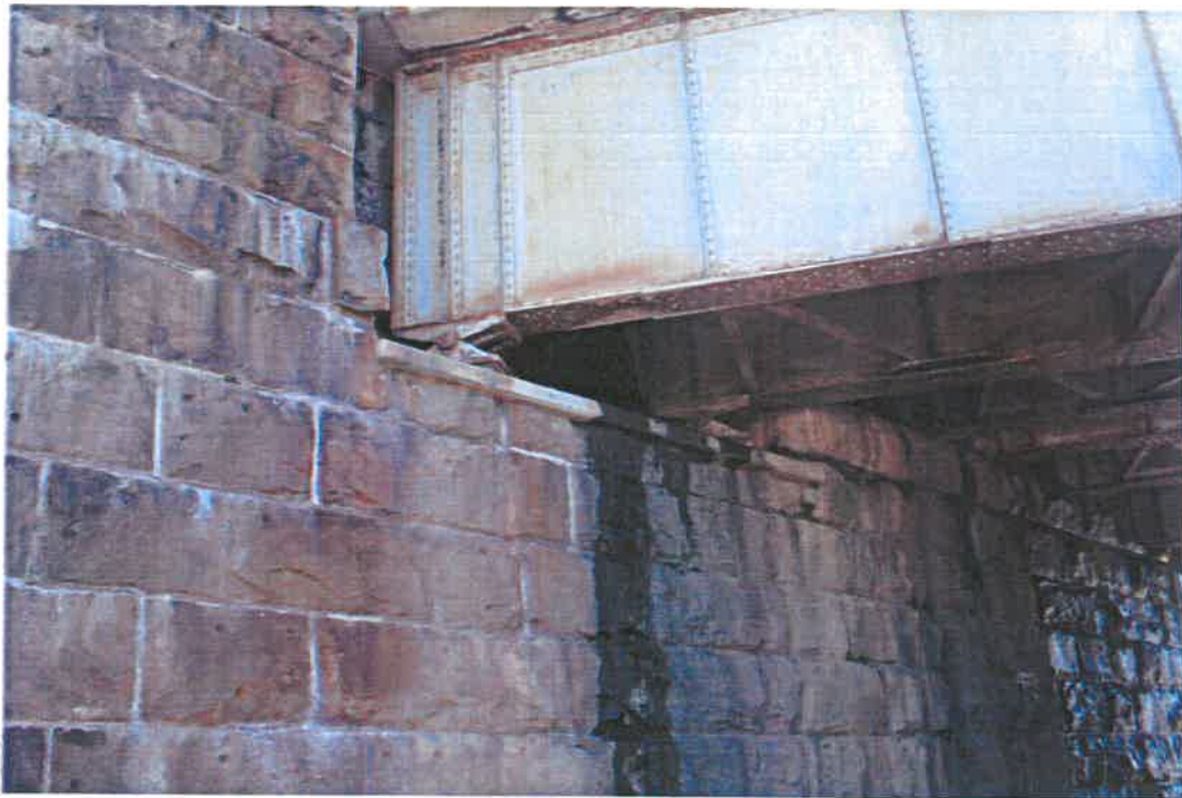
Abutment chop-down, capping & leakage at Juniata Street
