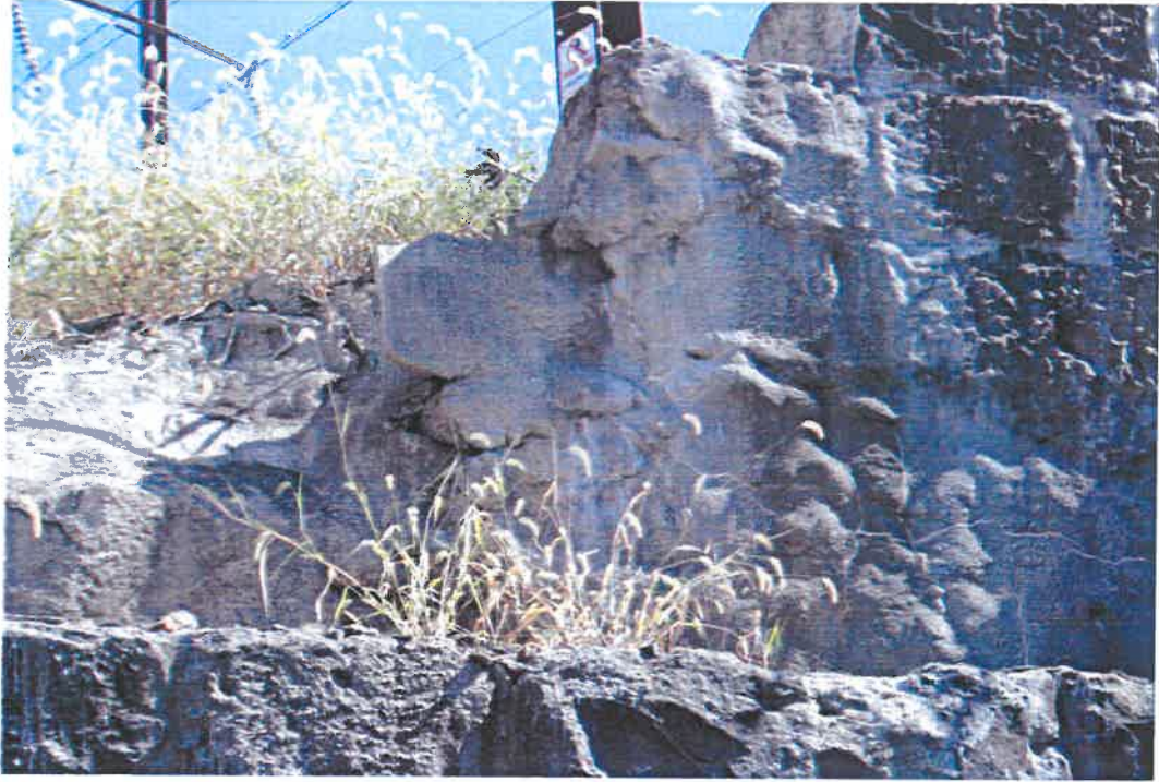
Severe abutment stone deterioration at Adams Street
