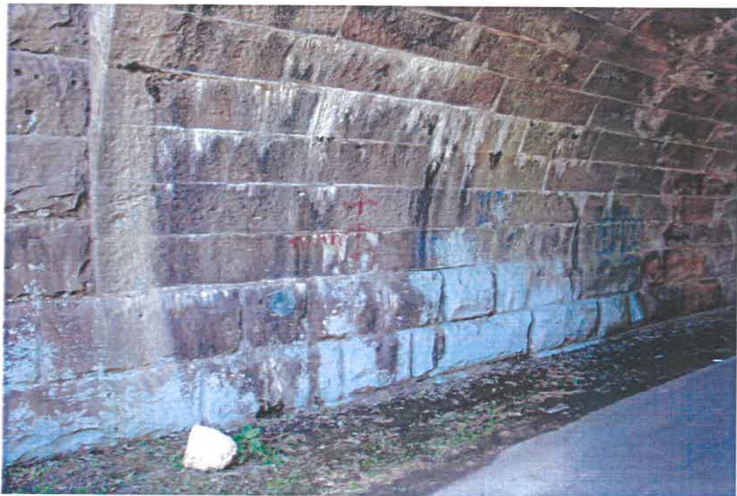
Leaching & discoloration within Centennial overpass
