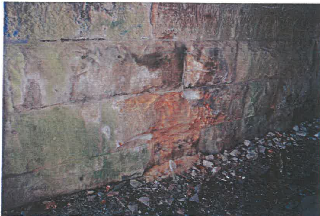
Leaching, discoloration & deterioration within Centennial overpass
