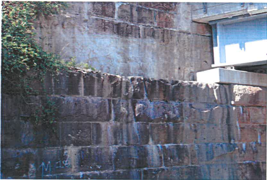
Patching & leaching at Adams Street
