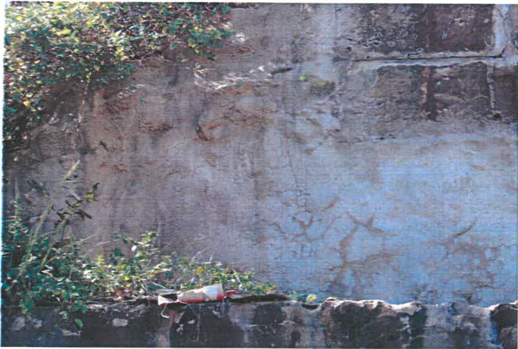
Deteriorated patching of chop-outs at Adams Street
