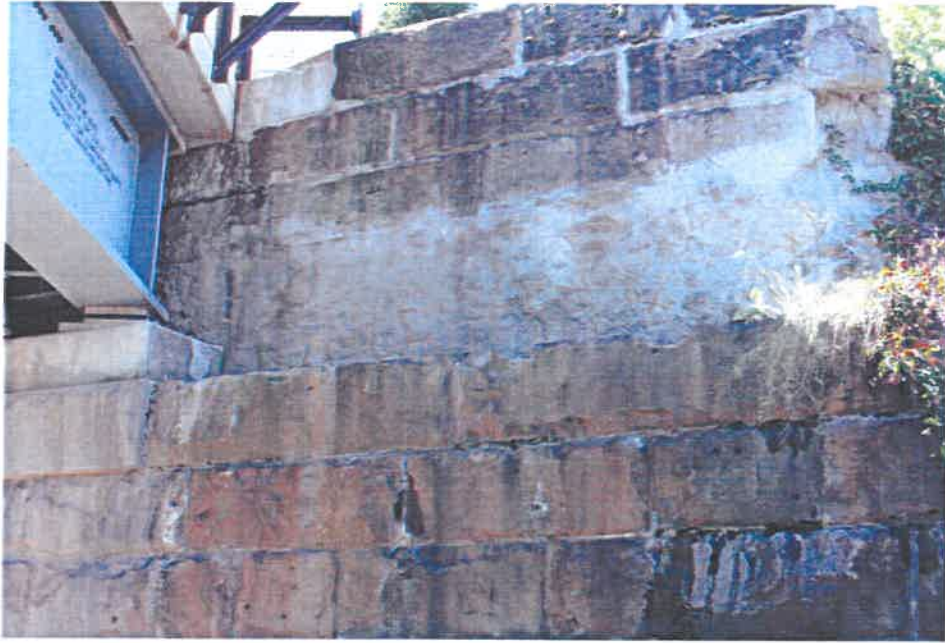
Unsightly, modifications & deterioration at Adams Street
