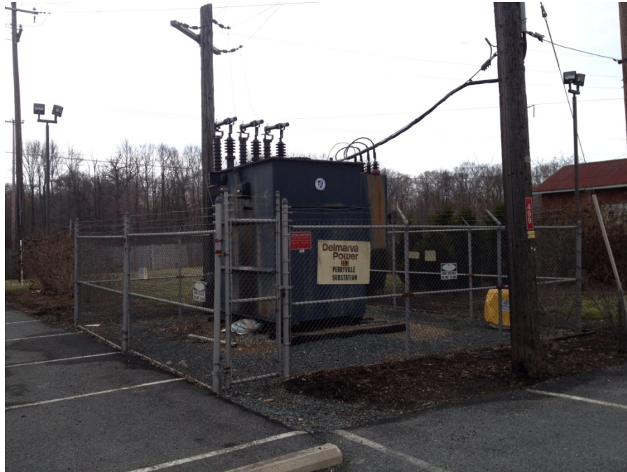
Electric substation on Perryville Post Office site, view to the southwest.
