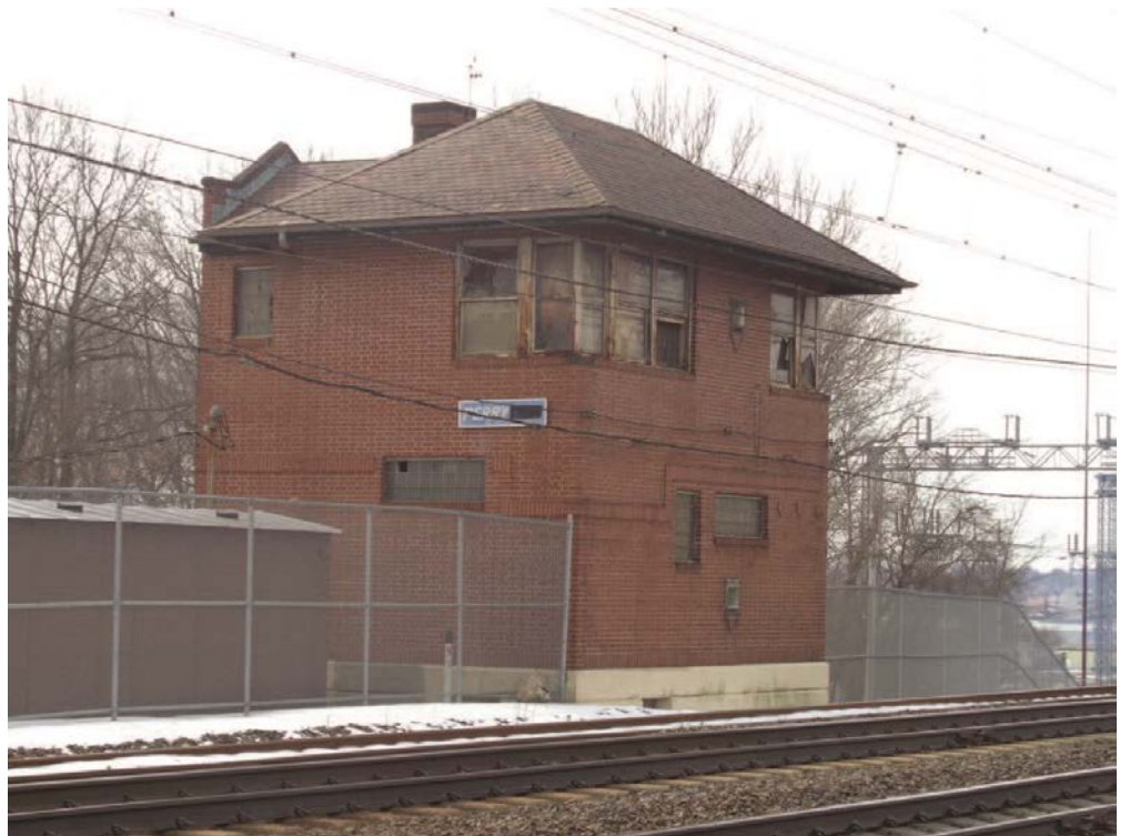
Perry Interlocking Tower: view of the north and east elevations; looking southwest. 22
