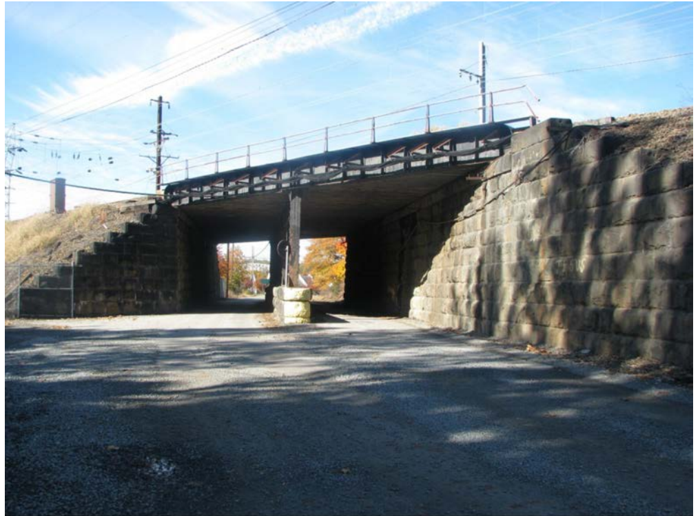
Access Road Undergrade Bridge (MP 59.52): View of the east side, which will be altered via replacing the existing concrete encased stringer and superstructure and will be extended with a concrete abutment; looking northwest. 27
