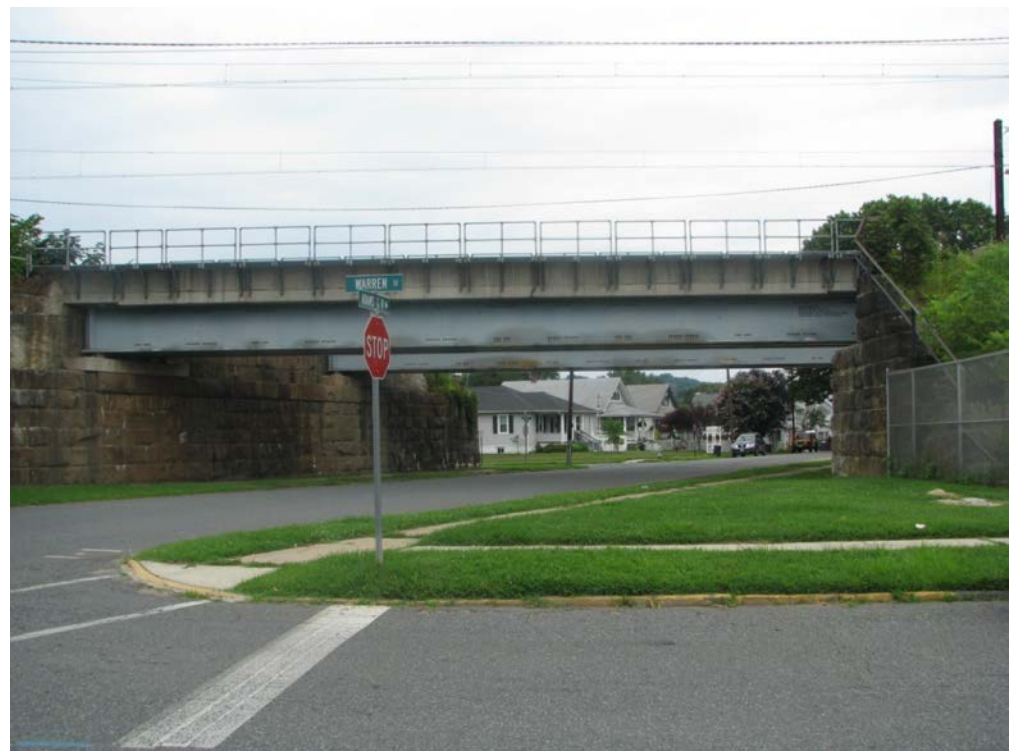
North Adams Street Undergrade Bridge (MP 60.69): view of the railroad east 14 side, which will be altered via construction of a new concrete abutment; looking north.
