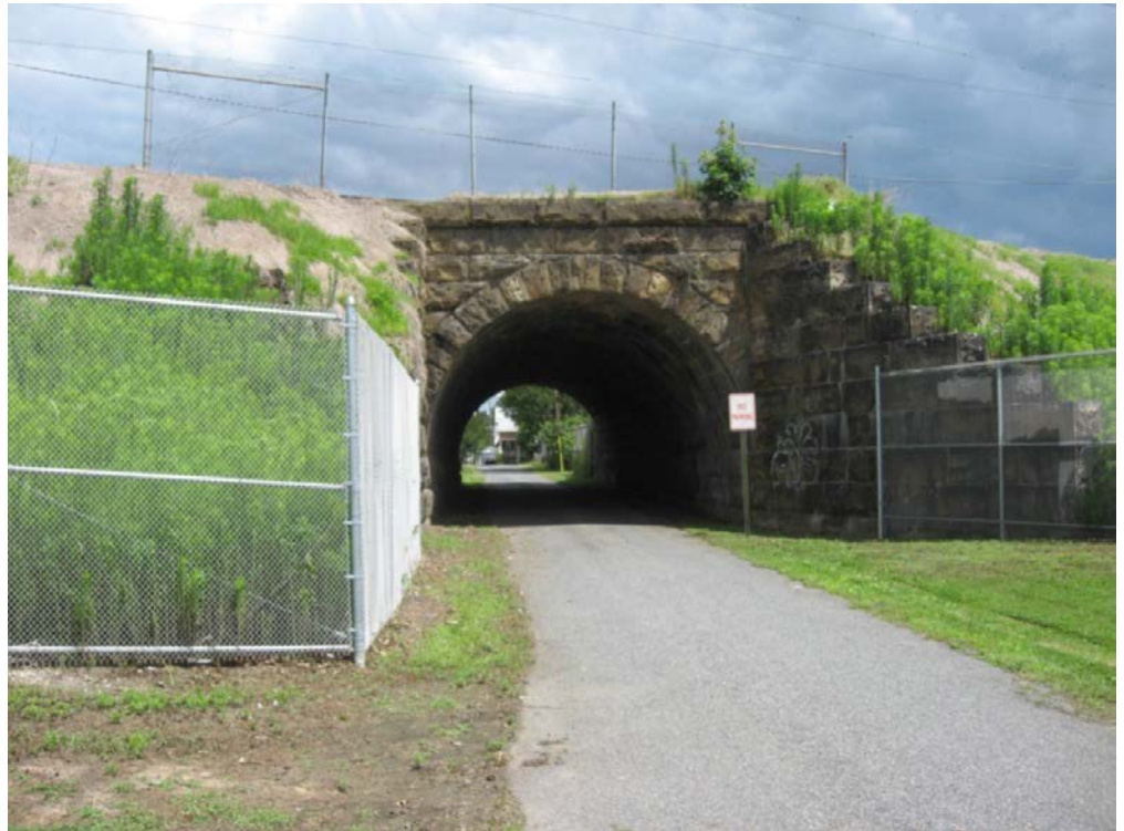
Centennial Lane Undergrade Bridge (MP 60.61): view of the railroad east side, 13 which will be altered via construction of a through plate girder bridge on a concrete abutment; looking north.
