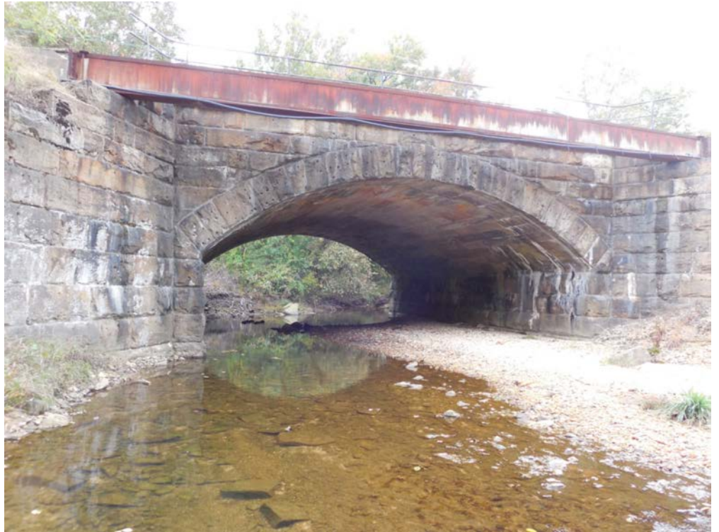
Mill Creek Undergrade Bridge (MP 59.00): View of the east side, which will be extended with a precast concrete culvert; looking northwest. 25
