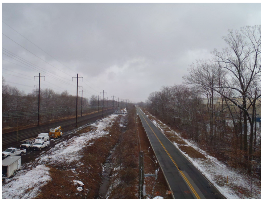
Photograph 12: General view of disturbed Amtrak ROW east of Firestone Road, facing east.
