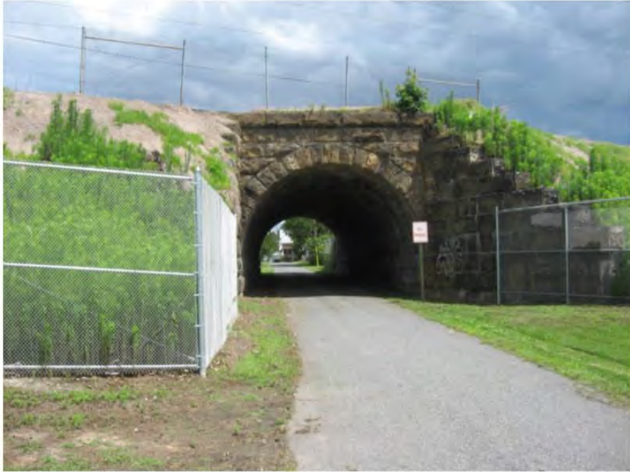
Photo 59: View looking north at the railroad east side of Centennial Lane Undergrade Bridge (MP 60.61), which will be extended with a precast concrete culvert and possibly altered via construction of a through plate girder bridge on a concrete abutment (for Alternate 9A only).
