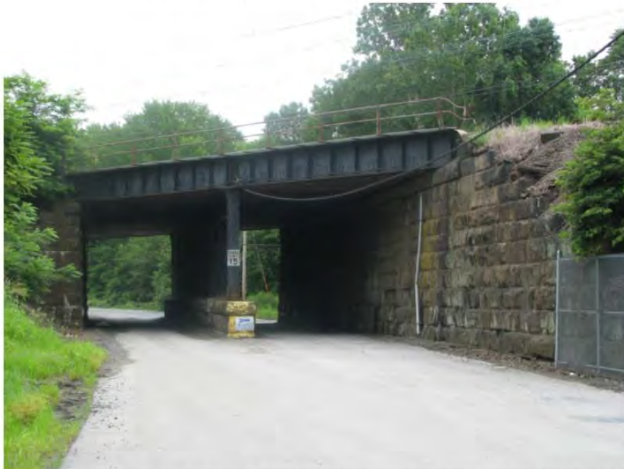
Photo 54: View looking southeast at the west side of the Access Road Undergrade Bridge (MP 59.52), which will be altered via replacing the existing structure with a precast concrete culvert (with a wider footprint) and partially demolishing and burying the abutments.
