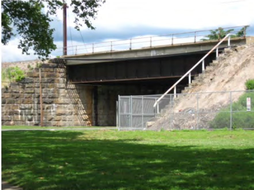
Photo 57: View looking northwest at the railroad east side of North Stokes Street Undergrade Bridge (MP 60.56), which will be altered via building a new concrete abutment.
