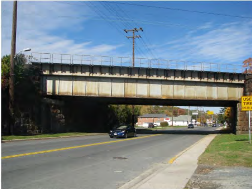
Photo 63: View looking northwest at the railroad east side of North Juniata Street Undergrade Bridge (MP 60.77), which will be altered via construction of a new concrete abutment.
