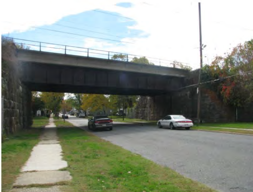
Photo 58: View looking south at the railroad west side of North Stokes Street Undergrade Bridge (MP 60.56), which will be altered via removing a portion of the existing stone masonry abutment and building new concrete abutment.
