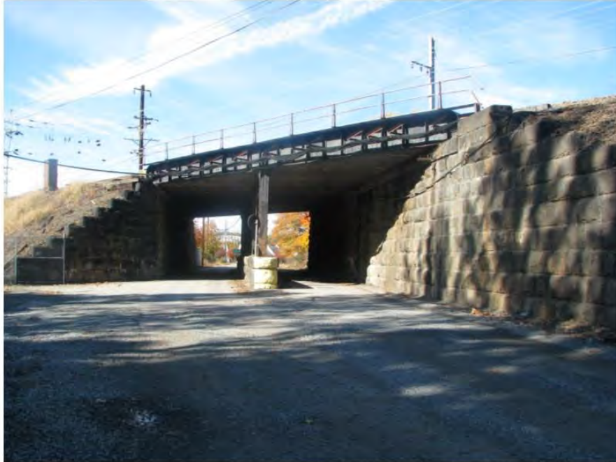
Photo 53: View looking northwest at the east side of the Access Road Undergrade Bridge (MP 59.52), which will be altered via replacing the existing structure with a precast concrete culvert (with a wider footprint) and partially demolishing and burying the abutments.
