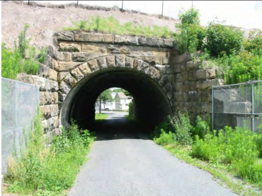
Photo 55: View looking north at the railroad east side of North Freedom Lane Undergrade Bridge (MP 60.51), which will be altered via construction of a precast concrete culvert.
