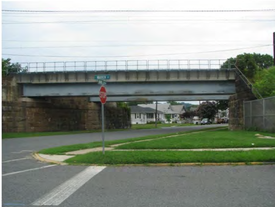
Photo 61: View looking north at the railroad east side of North Adams Street Undergrade Bridge (MP 60.69), which will be altered via construction of a new concrete abutment.
